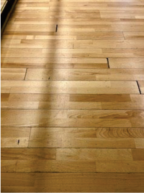
Gaps between floor boards.
