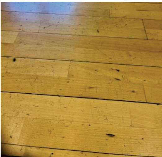
Separating floor boards and damaged wood.
