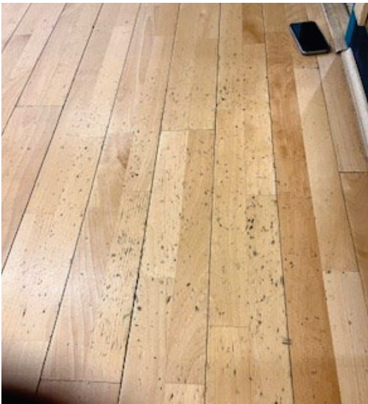
Marred floor with all floor boards separating.
