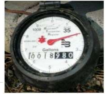
Water Meter Register
