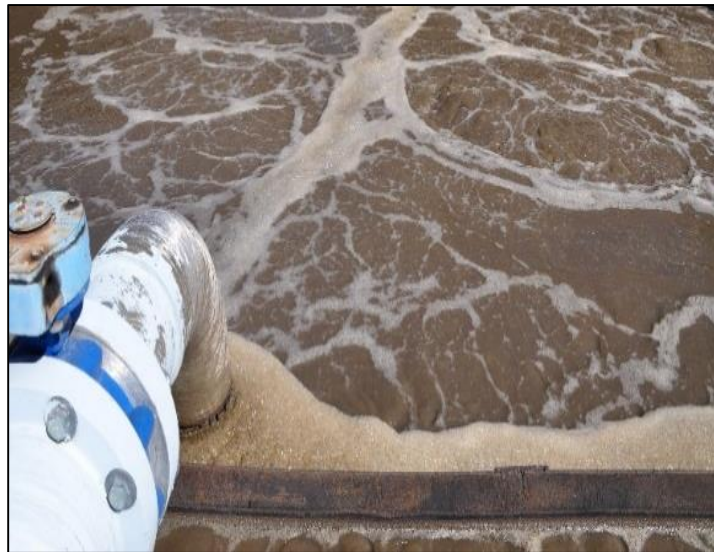
Aeration Process at the WRRF
