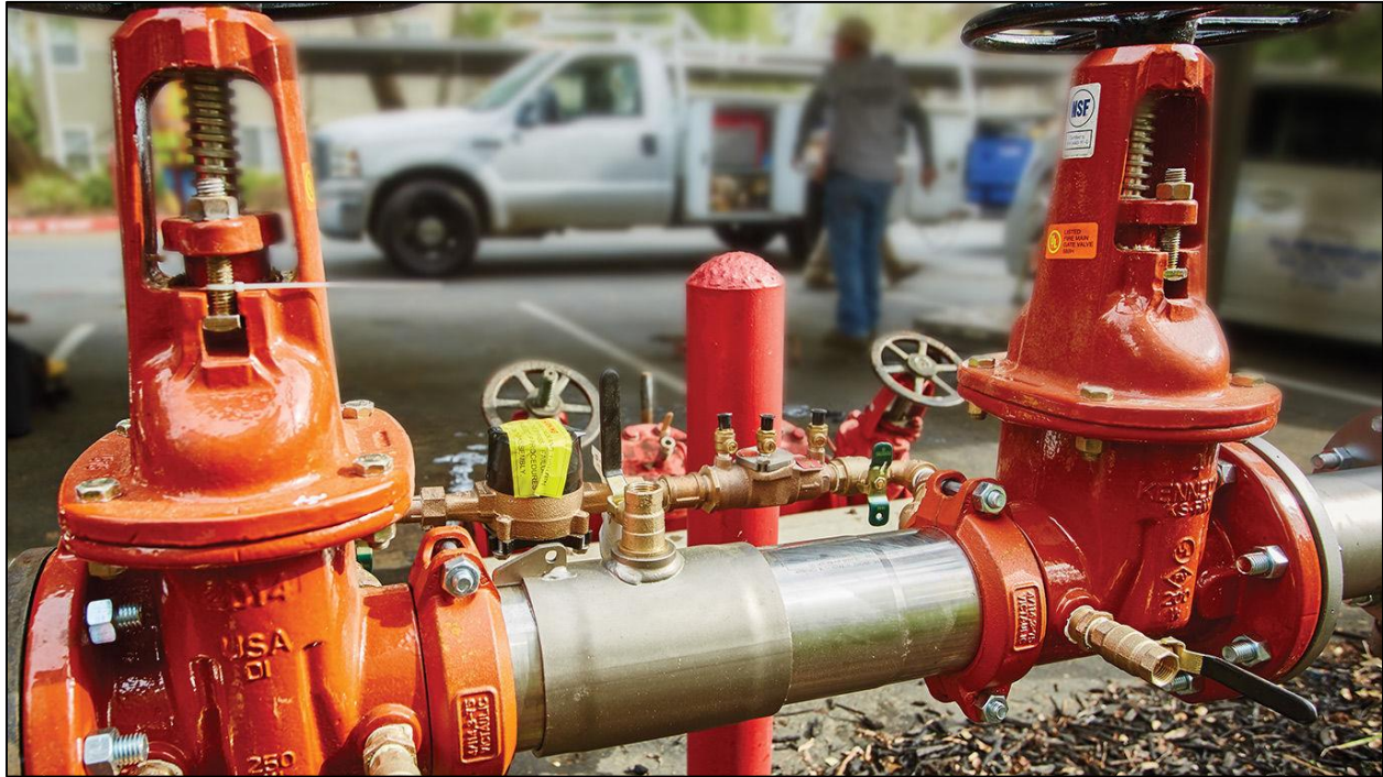
Backflow Prevention Device - Photo Courtesy of Watts (www.watts.com)
