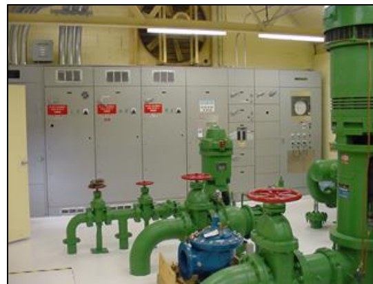
Spooner Pump Station
