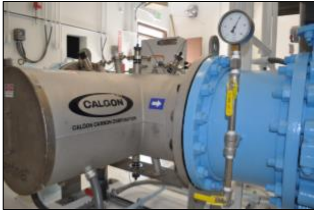
Chlorine Disinfection Chamber
