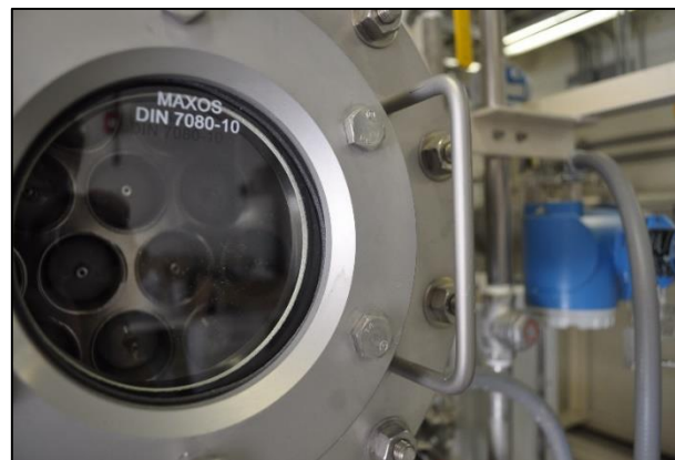
Drinking Water Disinfection Chamber
