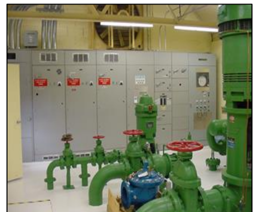
Spooner Pump Station
