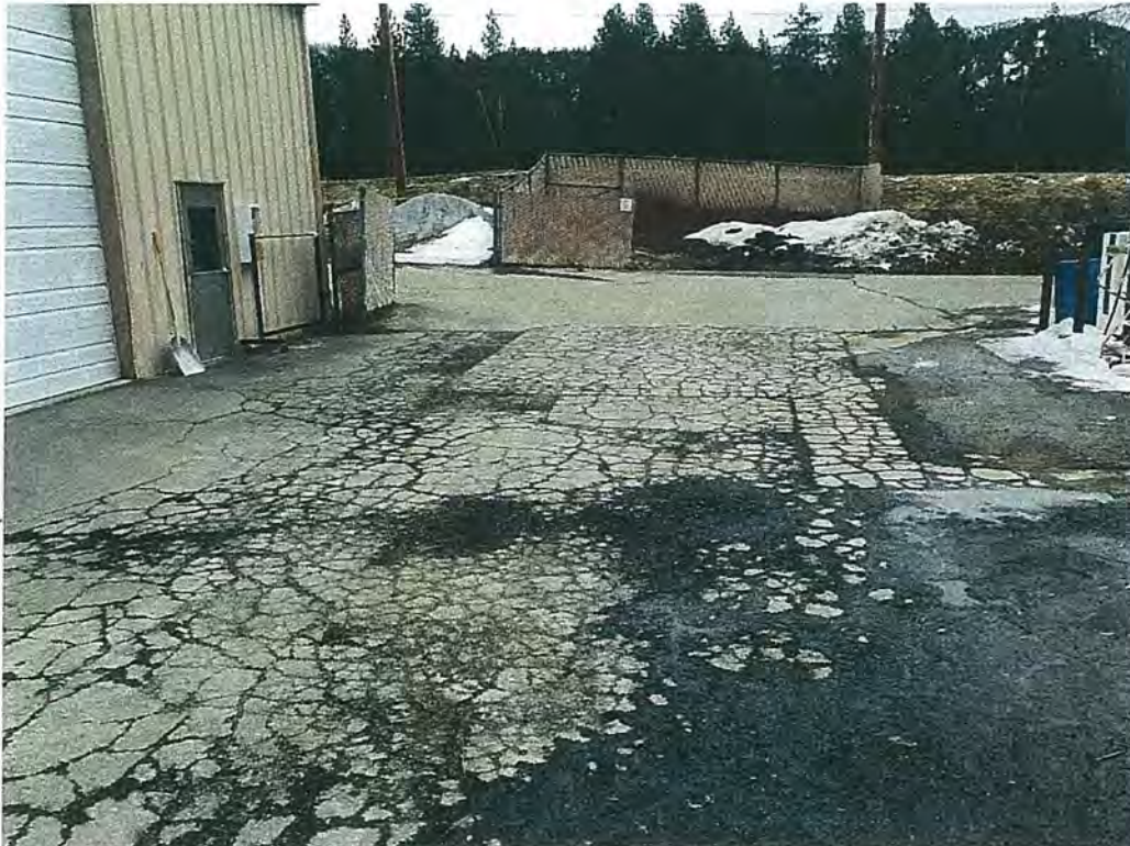
Photo 5. Deteriorated asphalt proposed to be replaced as part of a change order.
