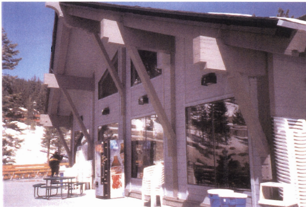
Existing conditions are carefully evaluated and compared with the needs of the community
