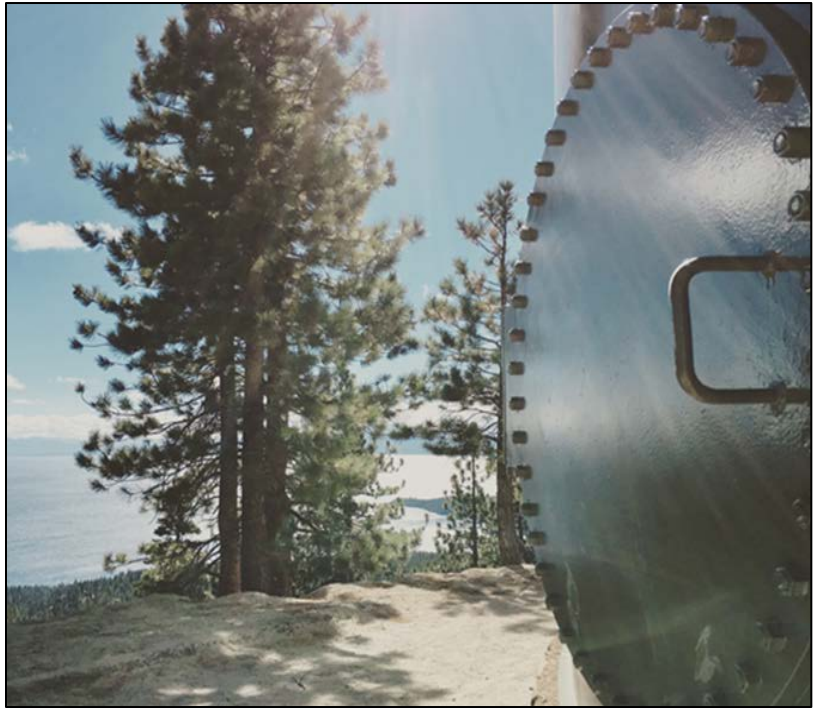
The upper-Tyner water tank (Reservoir 8-B1) is located at 7,771 feet in elevation and has a maximum drinking water capacity of 350,000 gallons.
