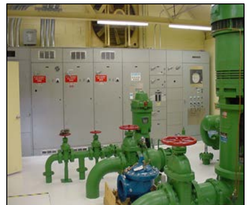
Spoooner Pump Station
