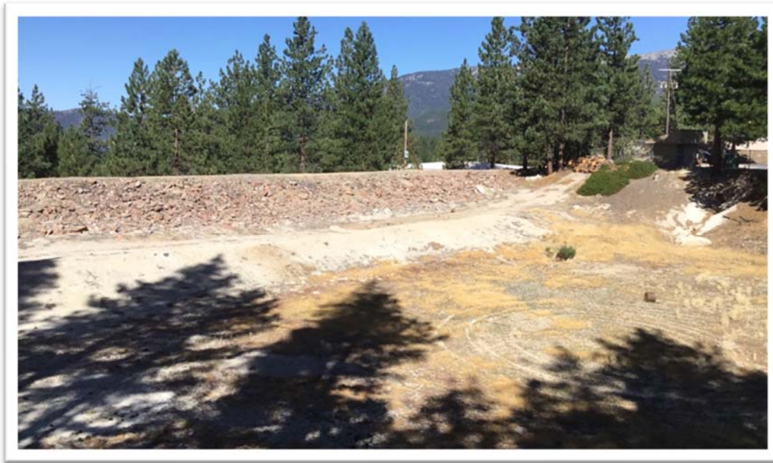
Figure 5. Overview of excavated unlined effluent storage basin (Pond #1). Dam to be removed and site regraded for tank foundation.
