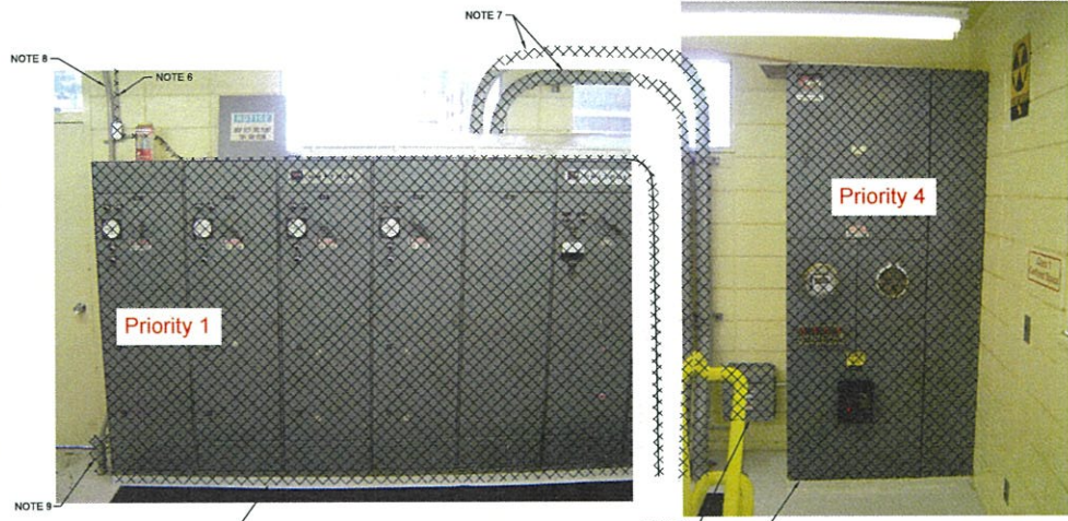
MCC-C LOOKING SOUTH WEST
