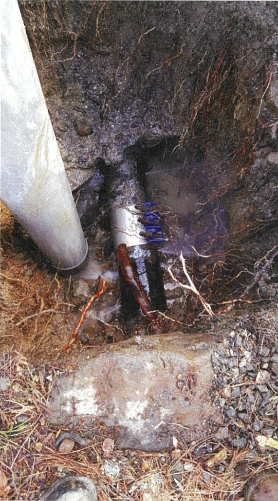
Photo of leaking waterline directly adjacent to a previous repair clamp.
