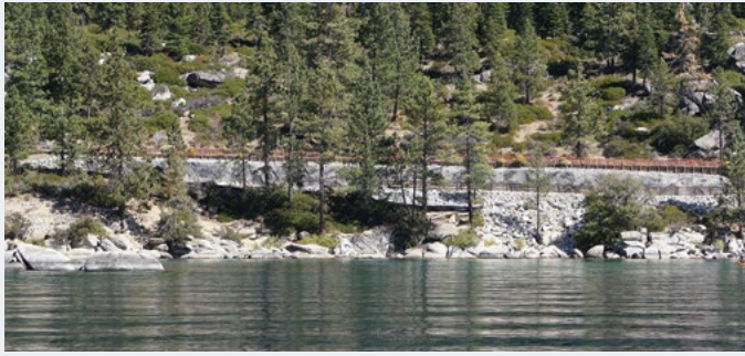
Approx. 2,400 lineal feet of soil nail wall sections now help stabilize the hillside.
