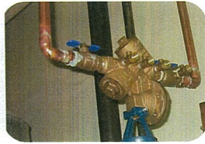
provide safe tap water.
