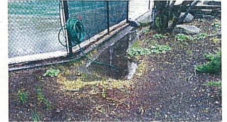
Site drainage system backup
