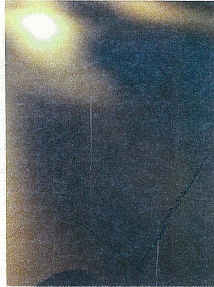
IVGID Courts #7-8 Repair and striation cracks
