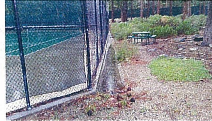
Site drainage backup
