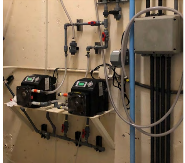
Figure 27: Chlorine Metering Pumps
