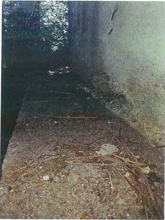
Photo 5 – Spalling at West Abutment Wall
