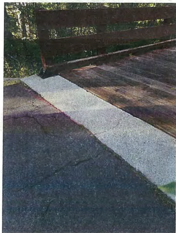
Photo 8 – Crack at East Abutment Approach Apron
