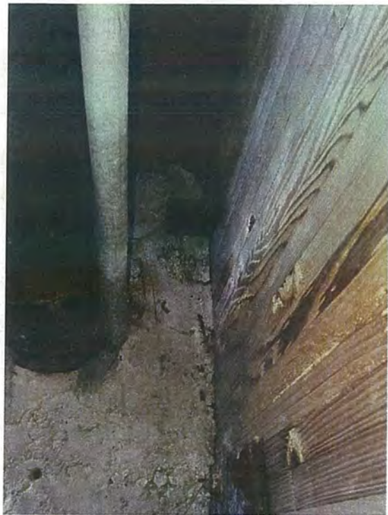
Photo 6 – Spalling at Top Connection Southwest Beam Bearing
