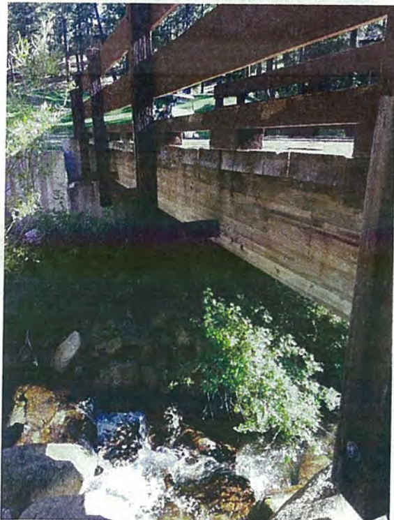
Photo 29 – Typical Weathering at Beams
