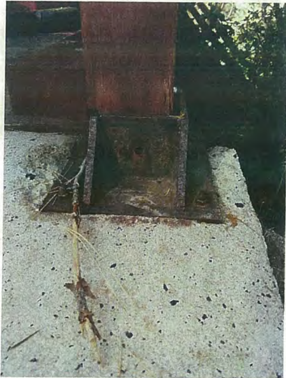
Photo 20 – Missing Bolt at End Post Connection
