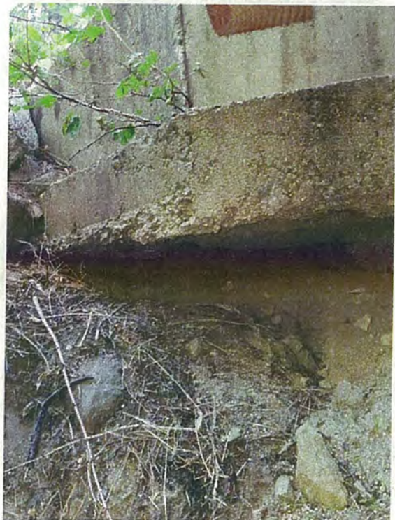
Photo 22 – Severe Scour at East Abutment
