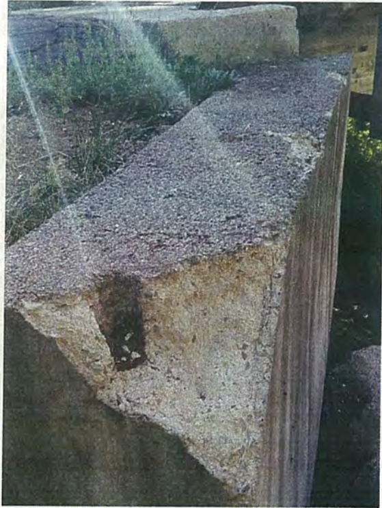
Photo 24 – Spalling at Northwest Wing Wall
