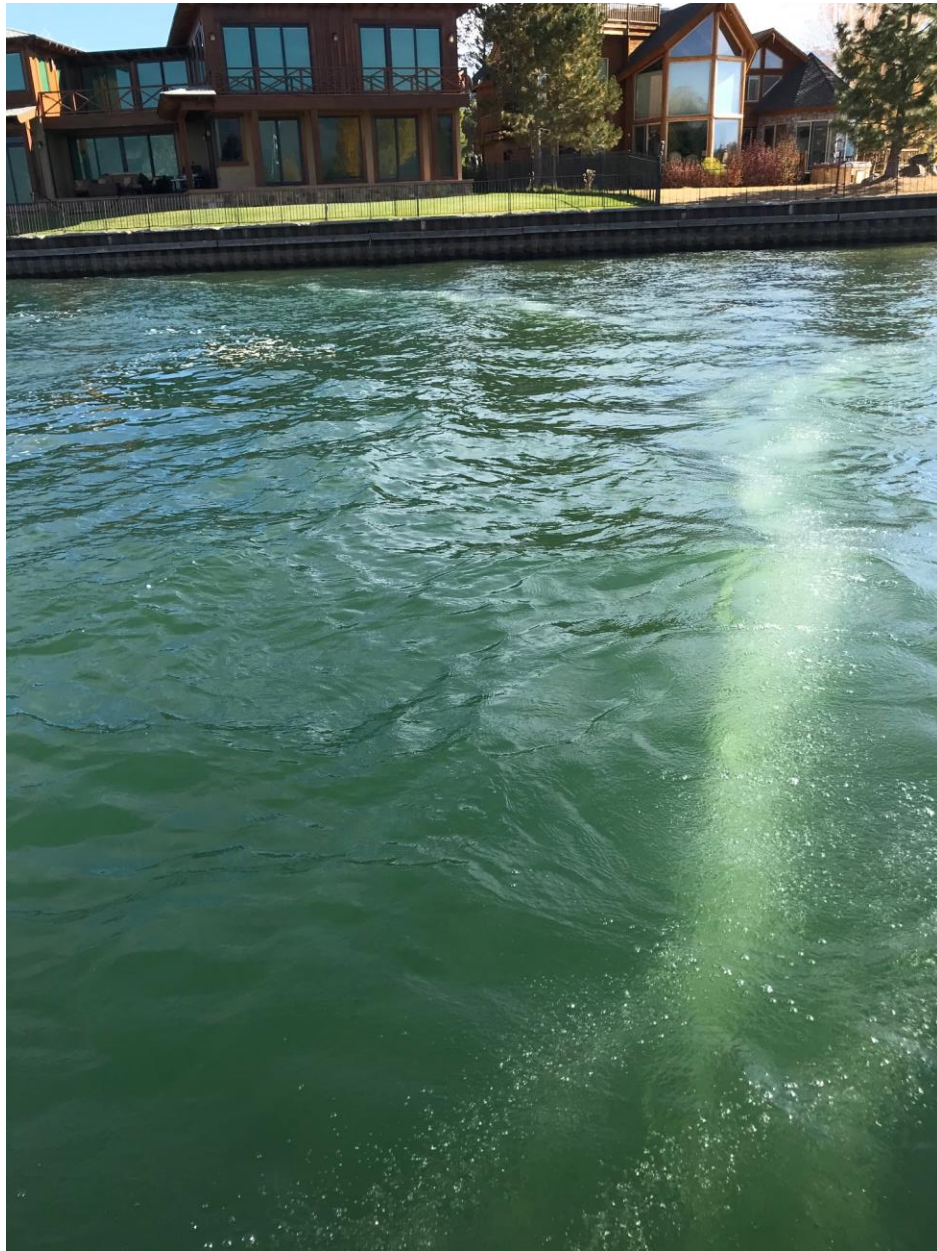
Fragment controlling bubble curtain - Tahoe Keys West Channel
