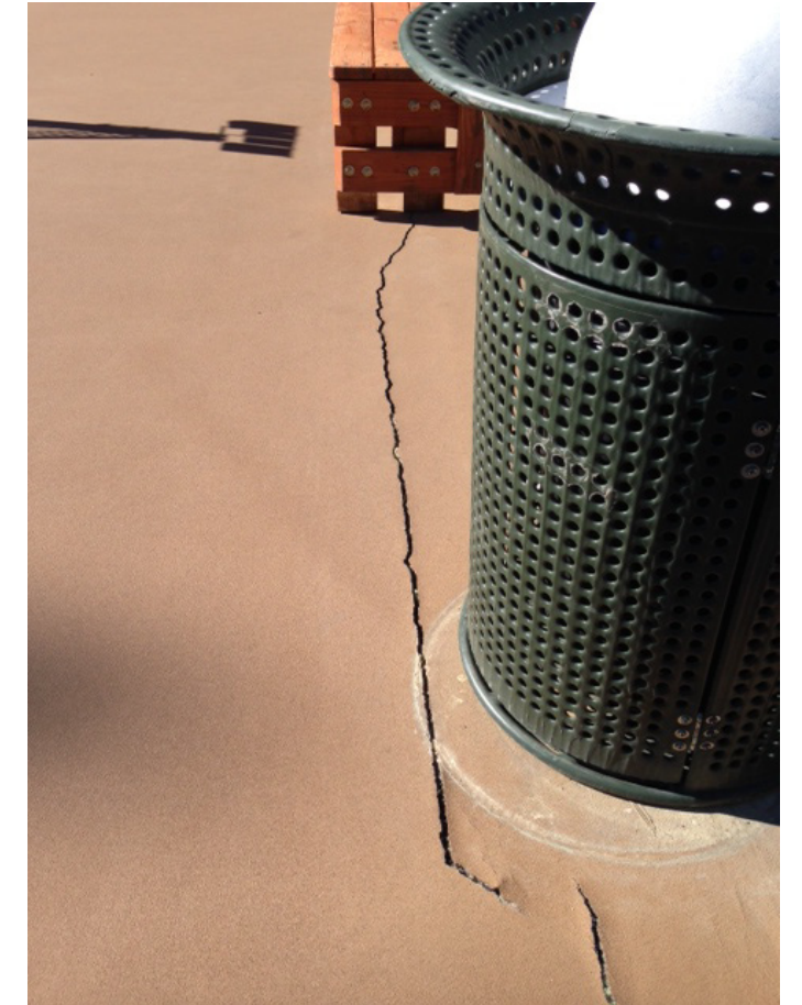
IVGID Courts #7-8 Surface cracking
