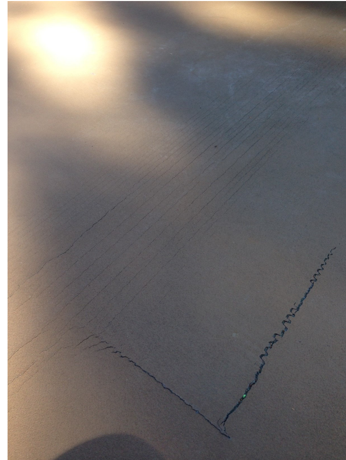
IVGID Courts #7-8 Repair and striation cracks
