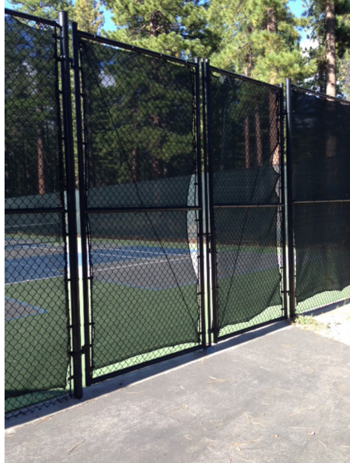
Gate with partial windscreen tears
