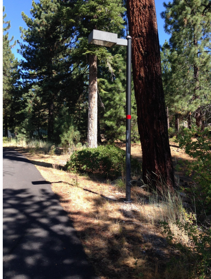
Main walkway lighting
