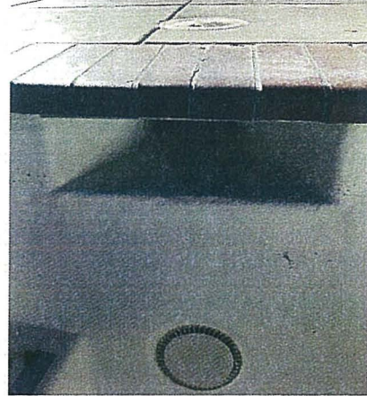
Pool Photo #2 Close-up of replacement pool skimmer. Note fiberglass finish and lack of waterline tile.
