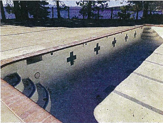
Pool | Non-compliant stairs noted.
