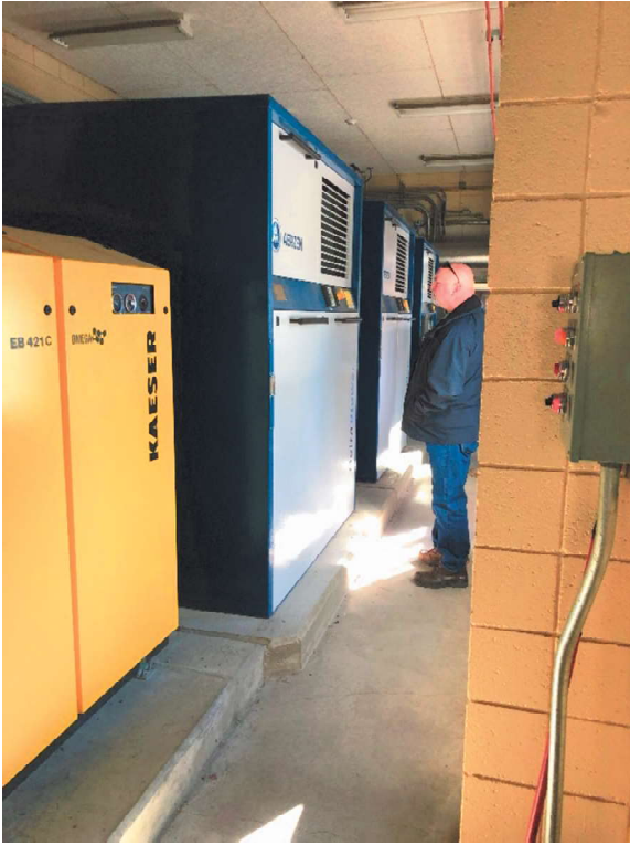
Figure 56: Aeration Basin Blowers and Blower
