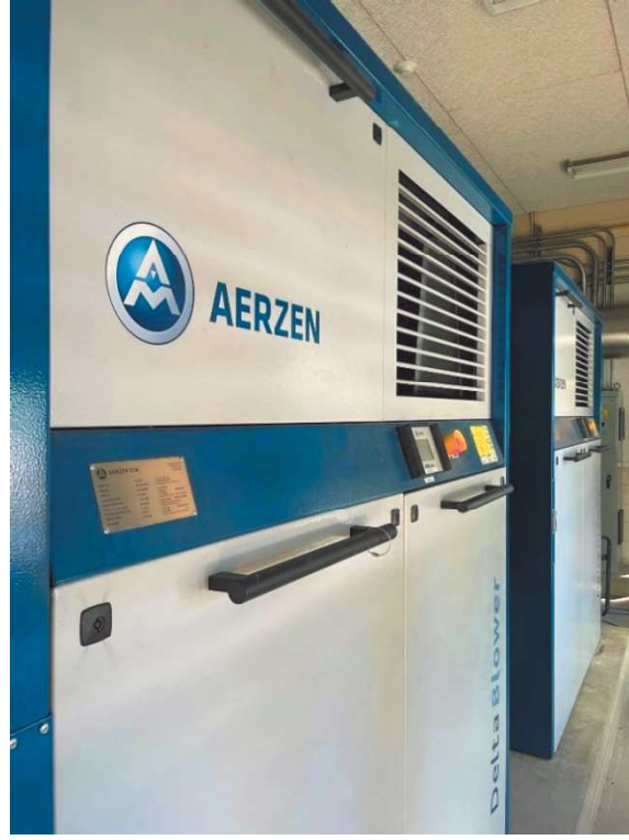
Figure 57: Aeration Basin Blowers/Enclosures
