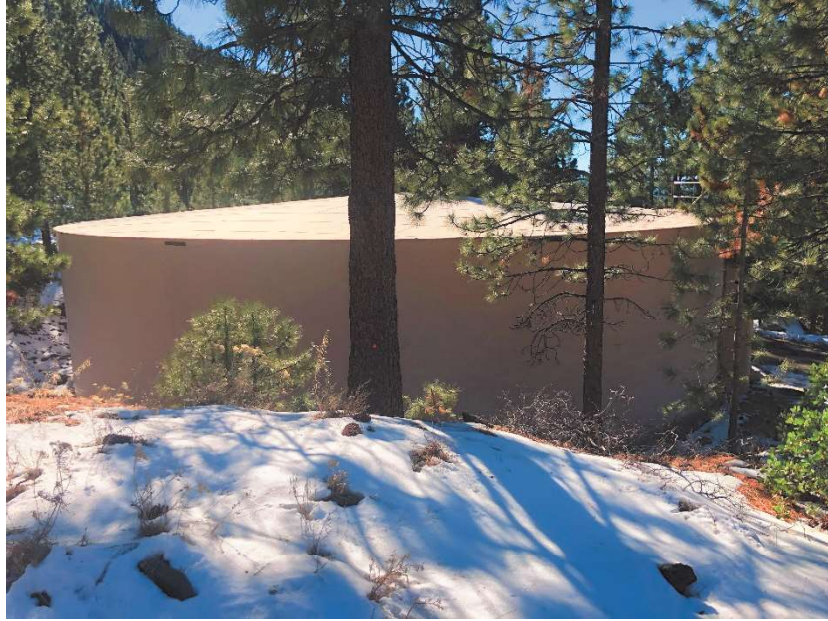
Figure 74: Effluent Storage Tank
