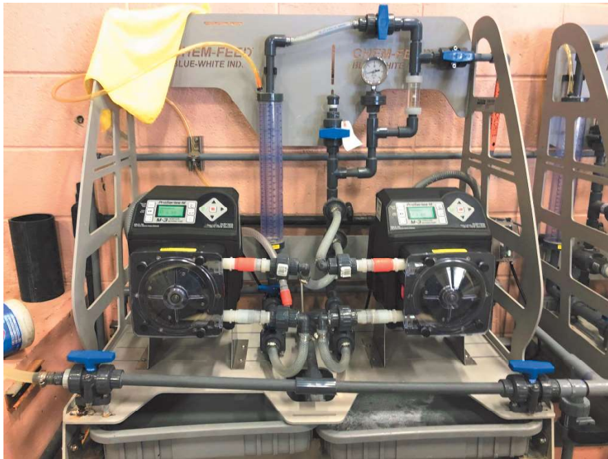
Figure 73: Hypochlorite Feed Pumps
