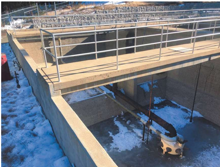
Figure 54: North Aeration Basin & “Jet Cluster” Diffuser, Empty (N-1)
