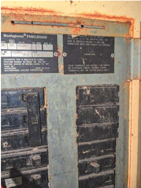
Figure 84: Panel Board Corrosion
