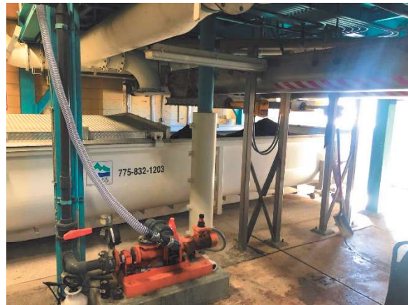
Figure 82: Polymer Transfer Pump and Sludge Cake Hopper
