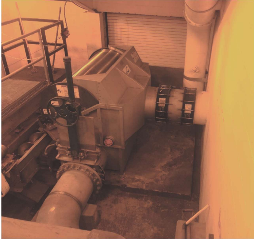
Figure 44: Headworks, Rotary Drum Screen (inlet/outlet)
