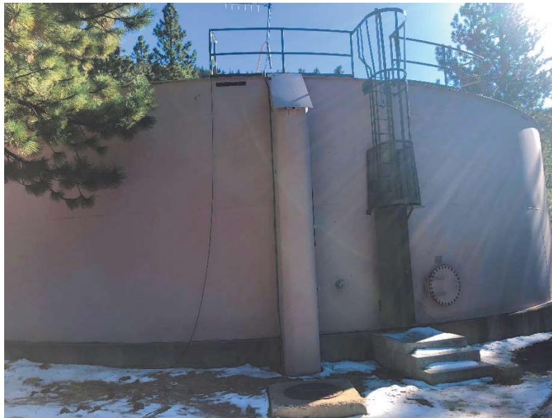
Figure 75: Effluent Storage Tank
