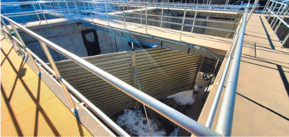
Figure 55: Aeration Basin, Anoxic Zone & Mixer (Basin S-2)
