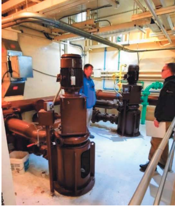
Figure 64: Return Activated Sludge (RAS) Pumps
