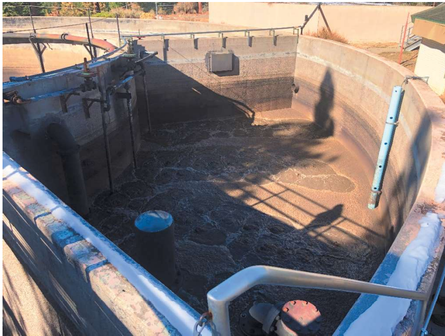
Figure 78: Sludge Holding Tank
