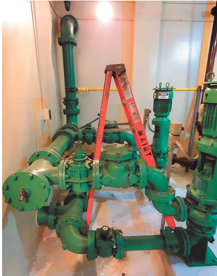
Figure 67: Plant Waste Pump Station
