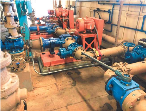
Figure 79: Sludge Pumps (Centrifuge Feed)
