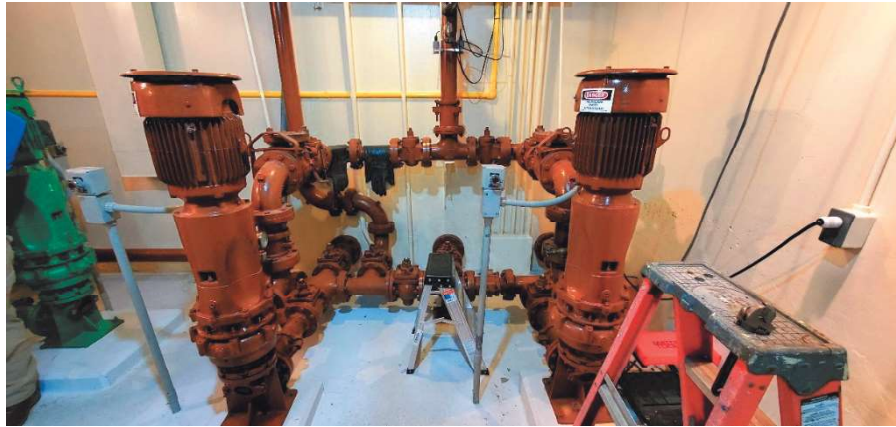
Figure 65: Waste Activated Sludge (WAS) Pumps
