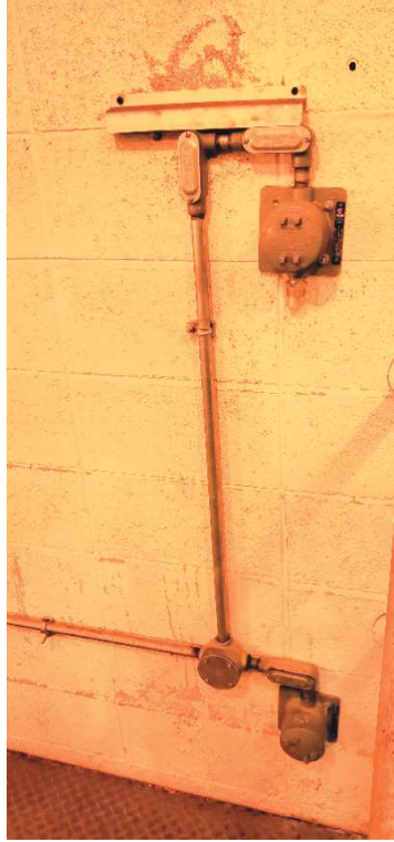
Figure 47: Hazardous Gas Monitor System Sensors (H 2 S & Low Oxygen)
