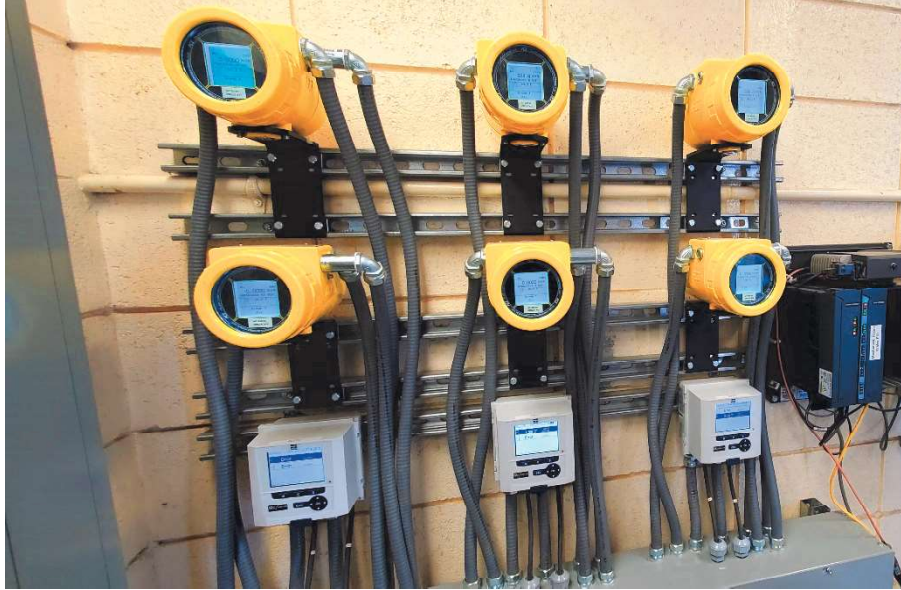
Figure 58: Dissolved Oxygen Monitors (3) and Mass Air Flow Meter Displays (6)
