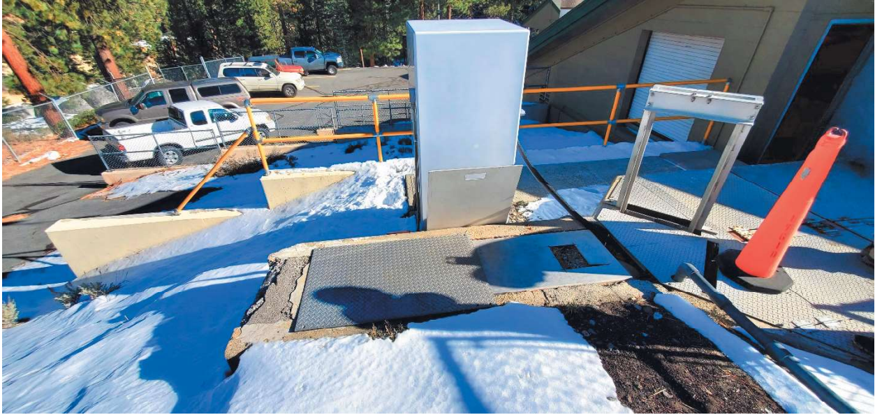
Figure 42: Influent Channels, Composite Sampler Weather Enclosure
