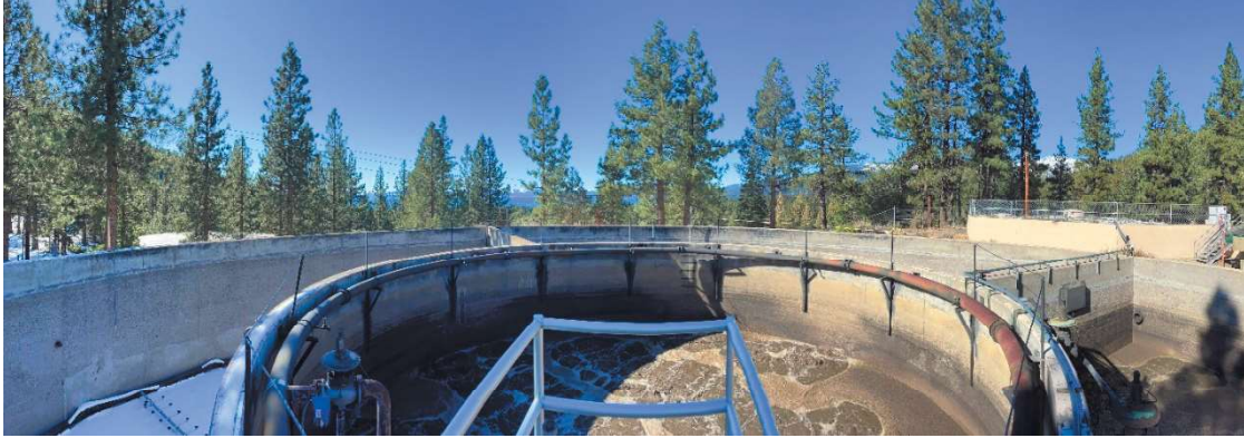
Figure 77: Center Sludge Holding Tank
