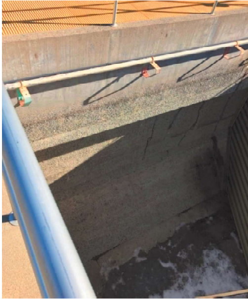
Figure 60: Aeration Basin Concrete Erosion
