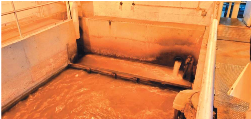
Figure 50: Grit Chamber & Outlet to Aeration Basins
