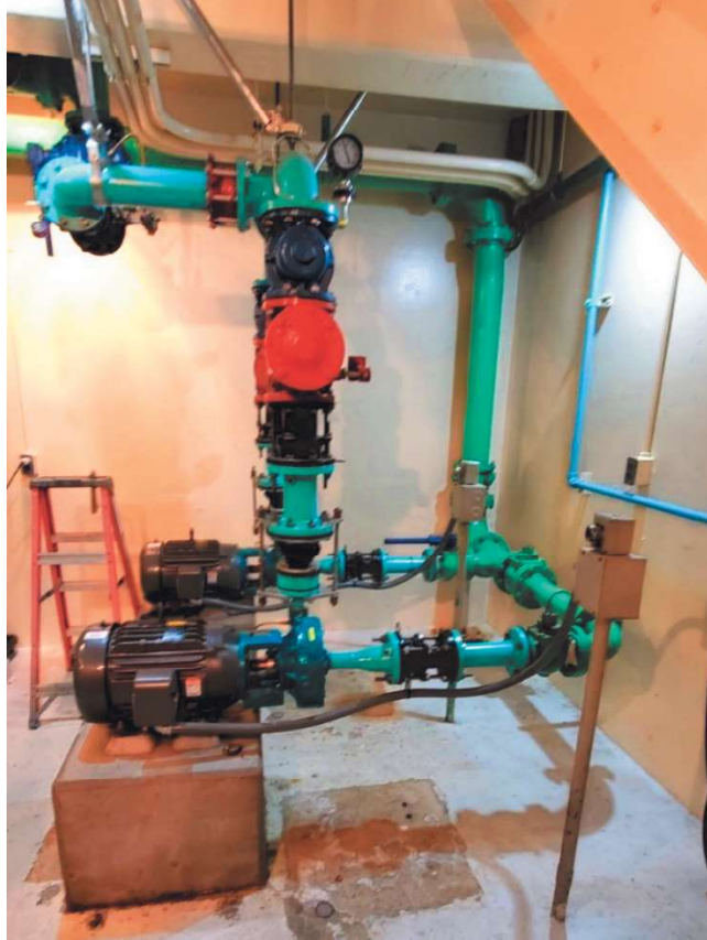
Figure 66: Plant Utility Water (non-pot) Supply Pumps
