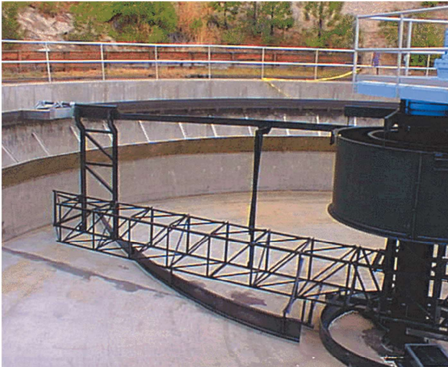
Figure 70: Secondary Clarifier Mechanism (example similar to IVGID)
