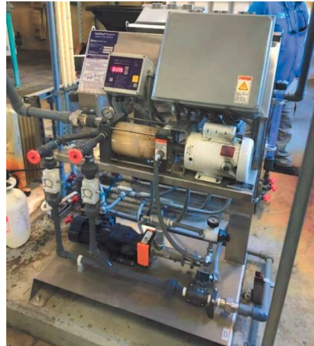
Figure 80: Dewatering Polymer Makeup and Feed System
