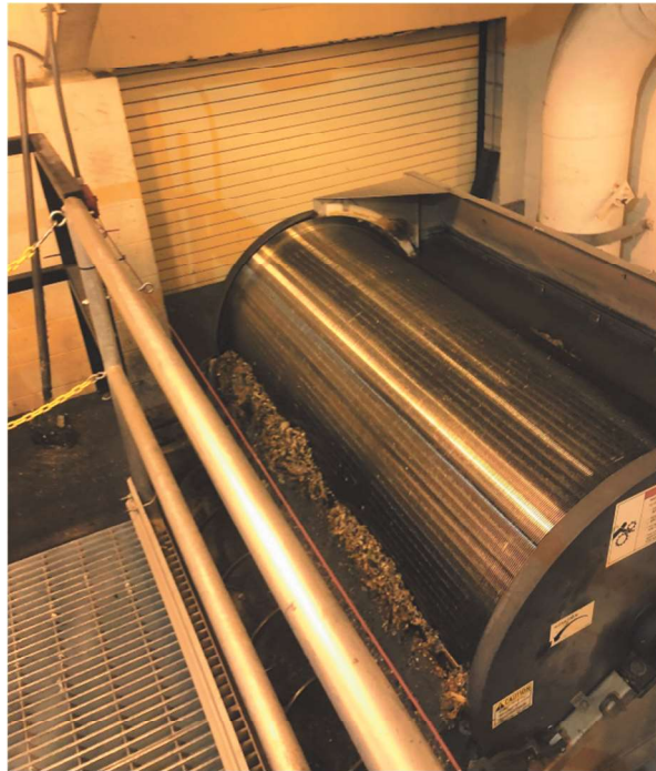
Figure 45: Headworks, Rotary Drum Screen
