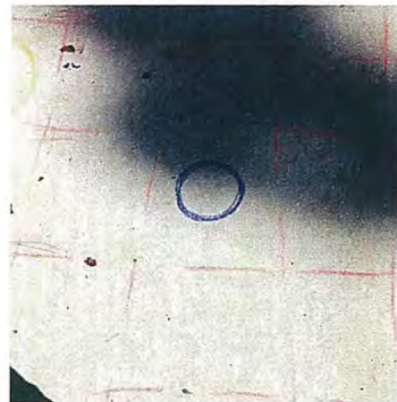
Pool Photo #6 Mapping of core location at swimming pool floor. Note additional mapping of rebar.
