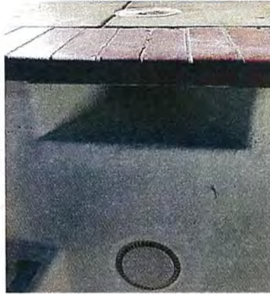
Pool Skimmer | Fiberglass finish and lack of waterline tile noted.
