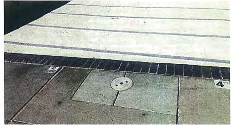
Pool Skimmer, Deck View | Limited deck replacement indicating limits of piping replacement noted.
