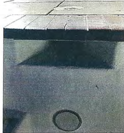
Pool Photo #2 Close-up of replacement pool skimmer. Note fiberglass finish and lack of waterline tile.
