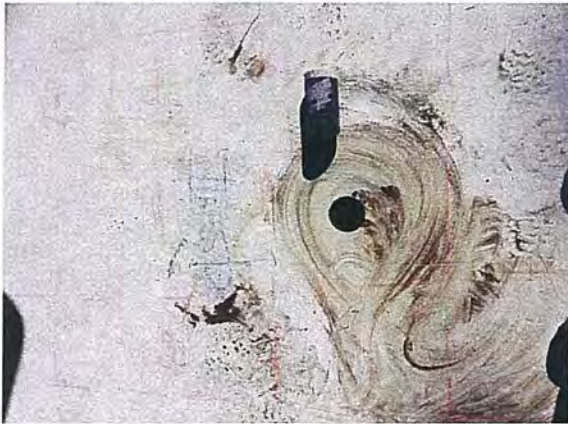
Pool Photo #9 Cored hole in swimming pool floor. Note, core sample for additional compression strength testing.
