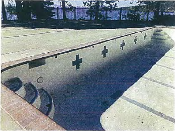
Pool Photo #1 South end of Pool. Note non-compliant pool stairs.
